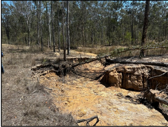
Plate 7: Area of erosion on eastern extent of the waterway through the north of Offset Area A.
