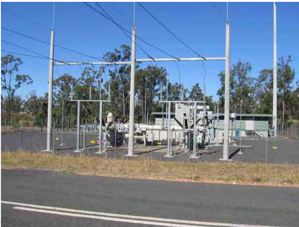
Figure 5 Energex Bulk Supply Substation
