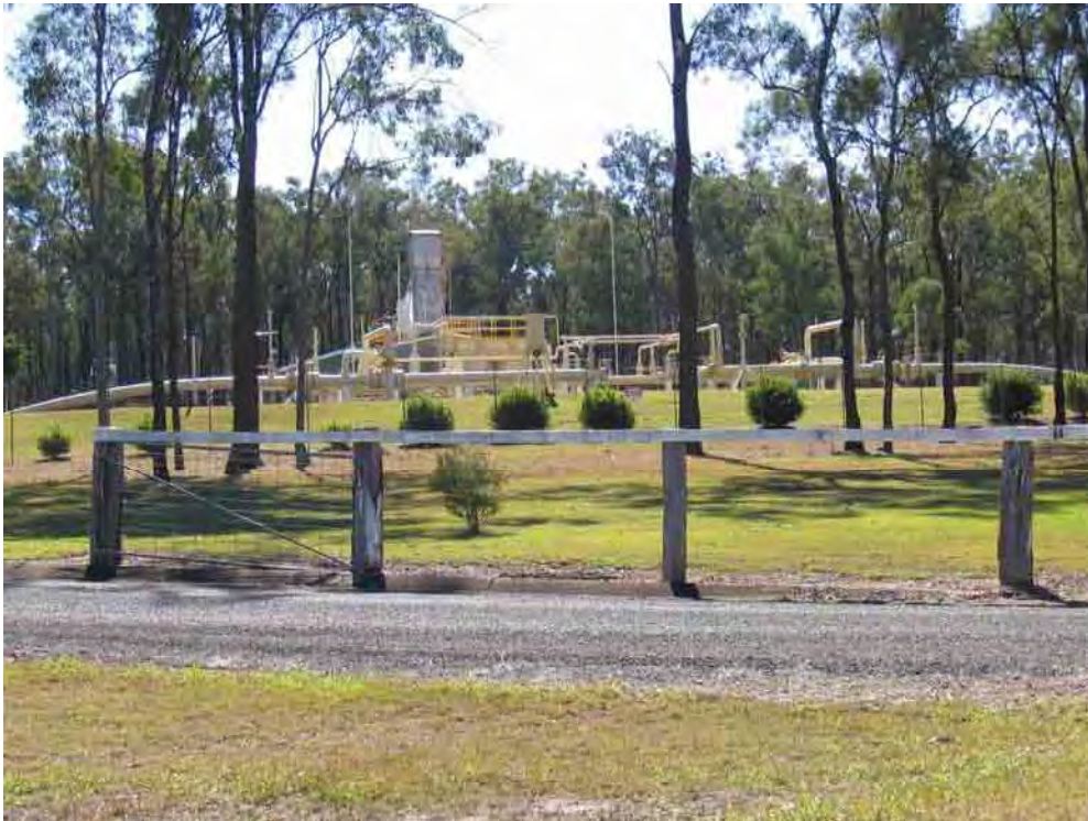
Figure 4 Gatton Gas Compressor Station
